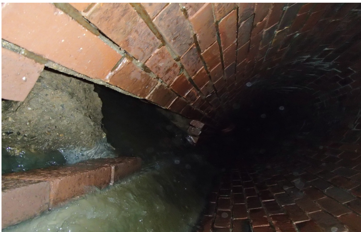
Fig. 7 – Visible damage to the sewer lining and a cavern between the Š1 and Š2 shafts (photo by INSET)
