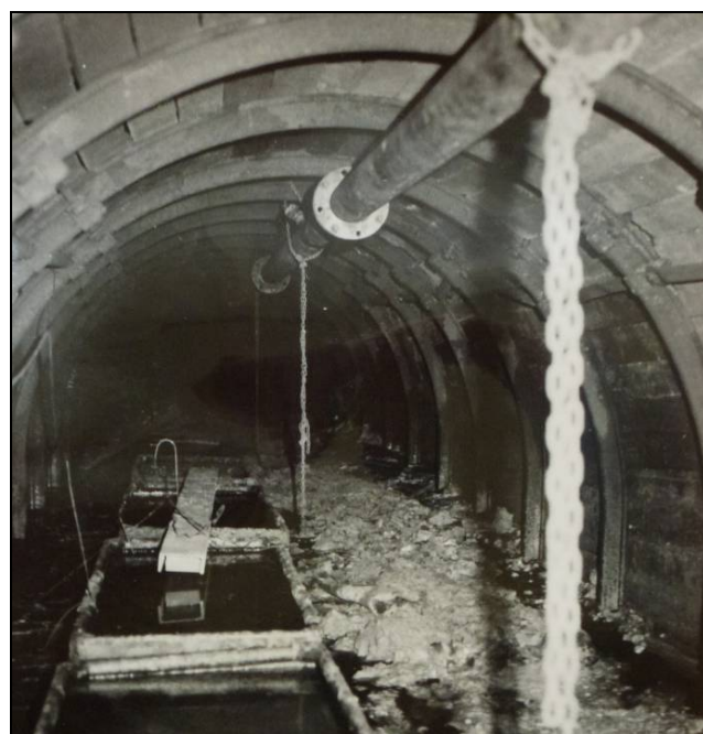
Fig. 4 – Photo of the fall in the fall of ground in the "P" sewer (2 July 1981), inrush created "tongue" – the flat cone reached the length of 140 – 150 m from the excavation face and even caved in the mining trucks
