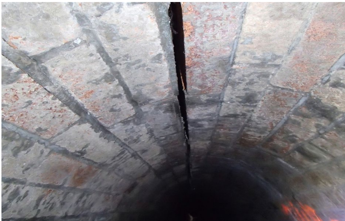
Fig. 6 – A visible wide-open longitudinal fissure (30 m long) in the sewer lining between the Š3 shaft and connection chamber (photo by INSET)
