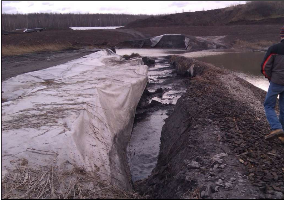
Fig. 3. Damaged earth dike.
