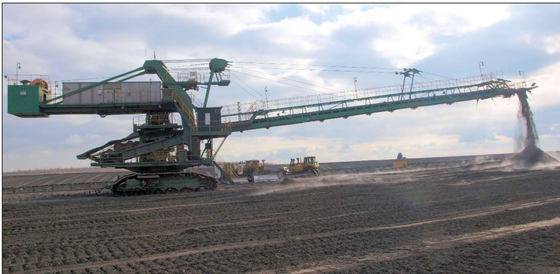
Fig. 1: Stacking the deposit material in the technical reclamation area using a belt stacker.
