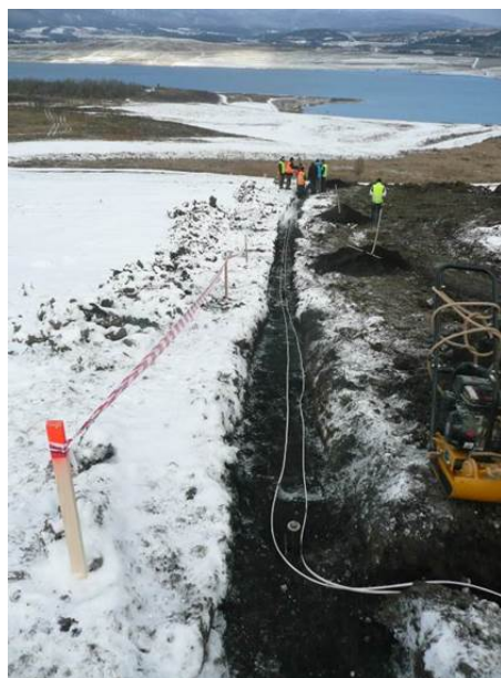
Instalace BOTDA ve svahu
